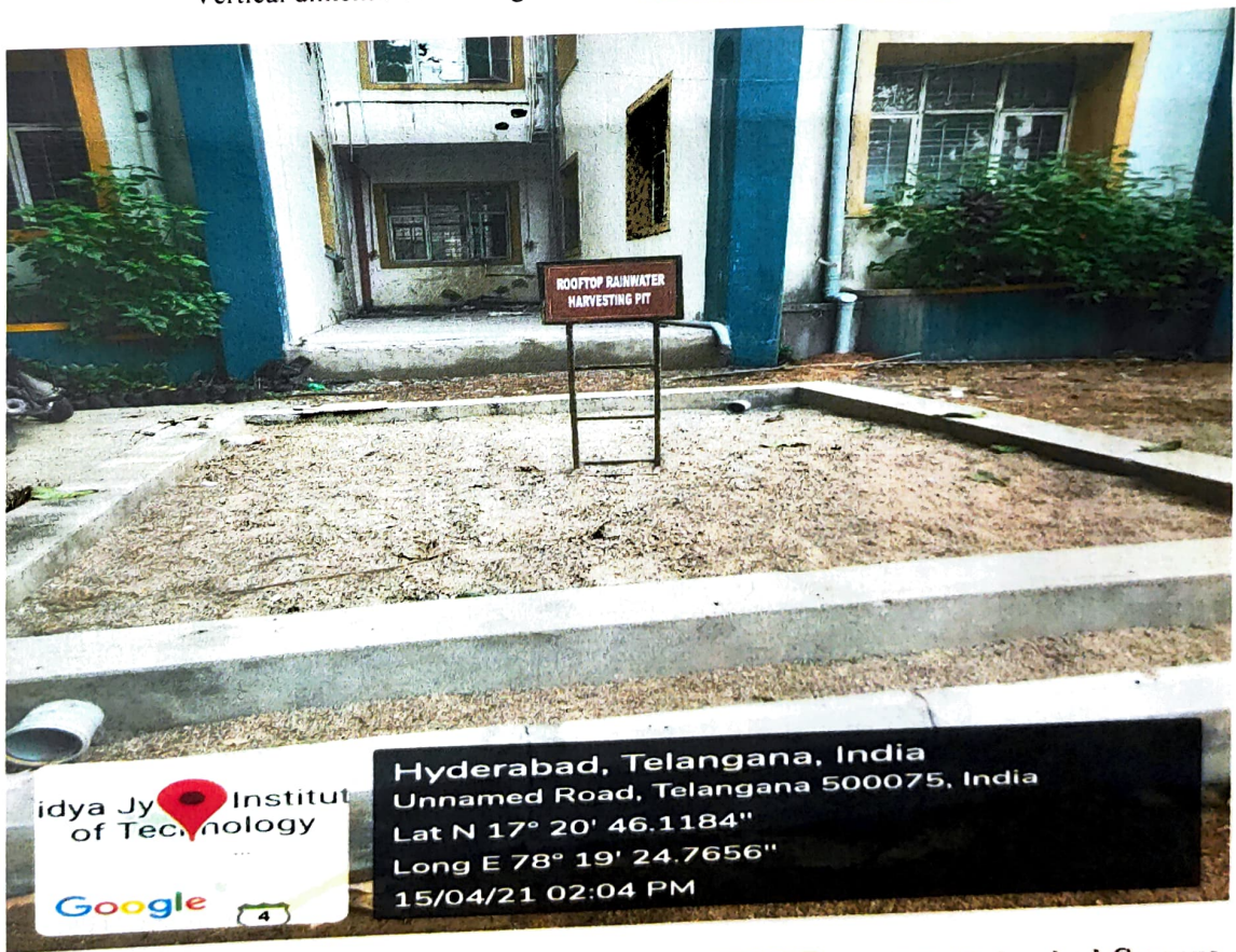
Roof top Rain Water Harvesting Pit of Size 10ft X 10ft X 8ft in VJIT, Hyderabad Campus
